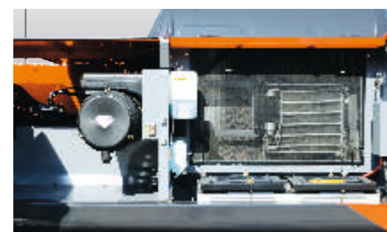
Utility space and radiators
